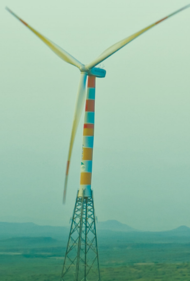
Nakhatrana Wind Farm, Gujarat, India
